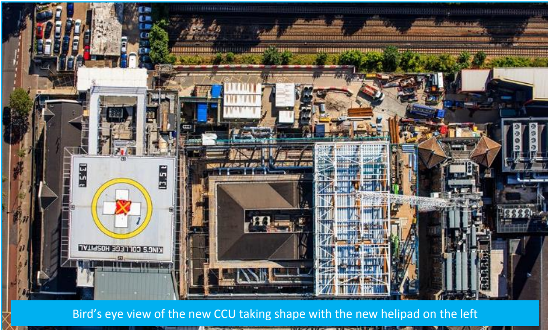
One of the seven sections being constructed above the theatre prior to pulling into place
