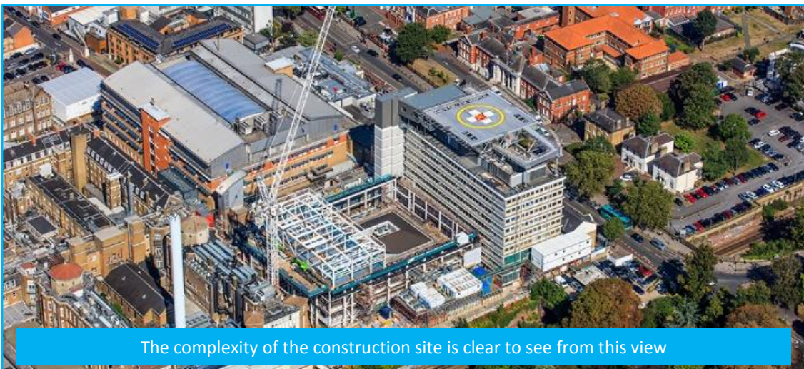
Bird's eye view of the new CCU taking shape with the new helipad on the left
